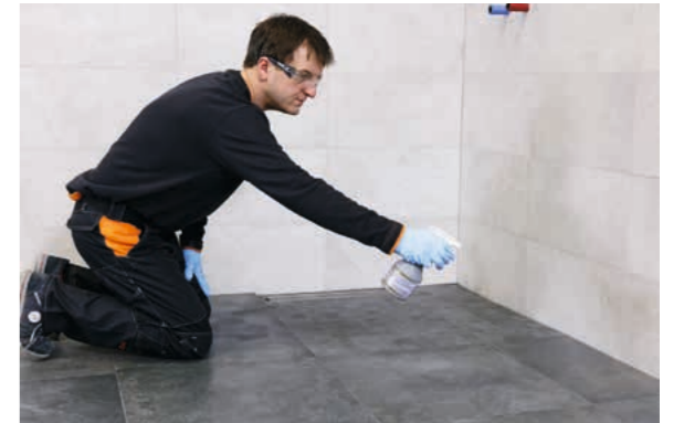
Before the final washing of the surface, PCI Durapox Finish (liquid) is sprayed onto the surface after about 60 minutes. Alternatively, PCI Durapox Finish (concentrate) may be added directly to the washing water.
