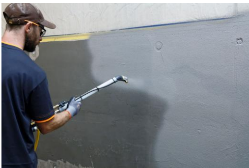
Application of PCI Barraseal Turbo 1K using the spray method ( Link to high-resolution picture ).
