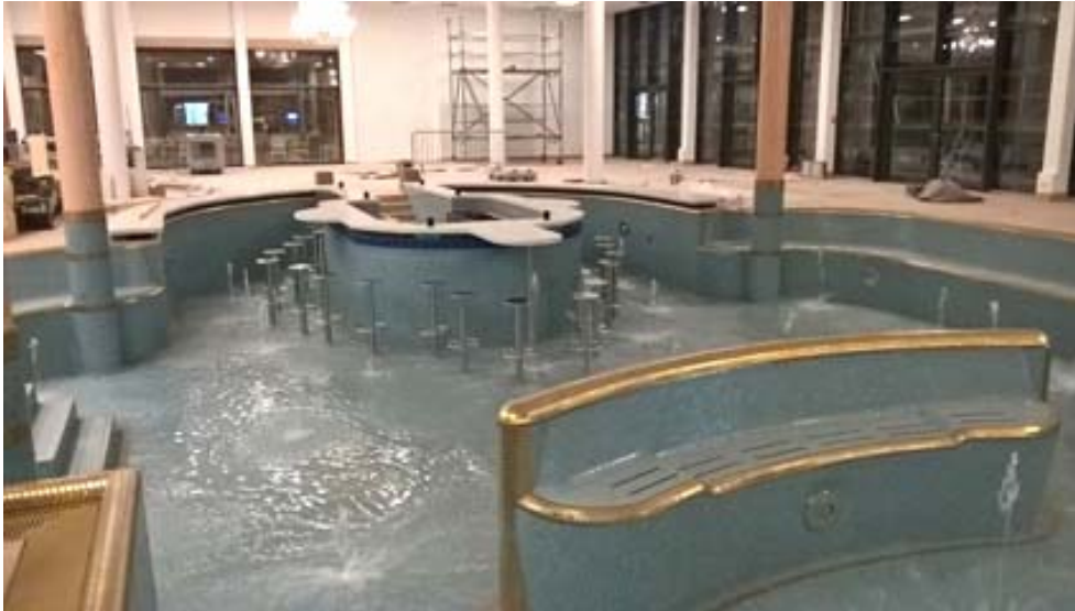
Fig. 11: Ready for the water. The tiling in the pool bar has been laid and grouted. Thanks to PCI Seccoral 2K Rapid, the substrate is absolutely watertight.
