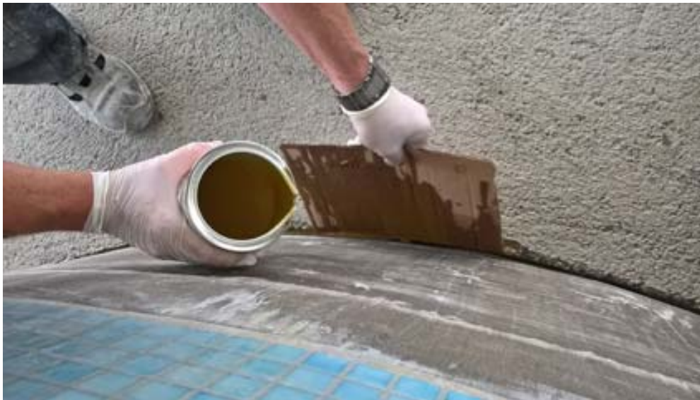
Fig. 6: Elastic grouting between the screed and the rising wall in the pool with PCI Apogel E.
