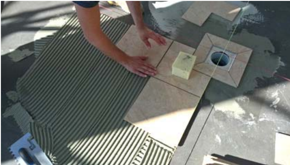
Fig. 9: The anti-slip tiling on the pool surrounds and in showers and changing rooms was laid using PCI FT Klebemörtel thin-bed adhesive with PCI Lastoflex polymer-modified additive.
