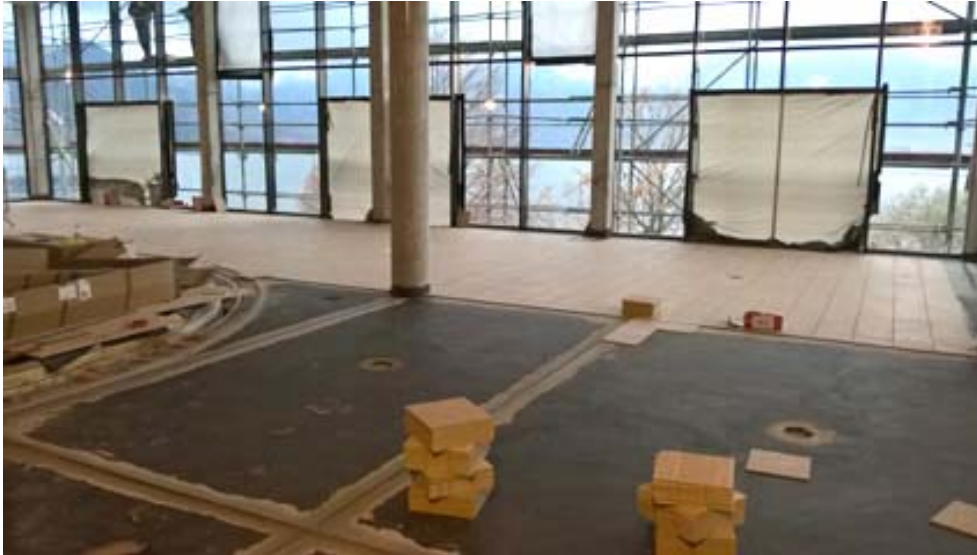
Fig. 10: The mosaic tiling of the pool was laid using PCI Durapox NT plus. This reaction resin mortar is especially well-suited for tiling exposed to chemicals, is wear-resistant, strong and insensitive to attack by swimming pool chemicals. PCI Durafug NT special cementitious joint grout was used for the pool surround.
