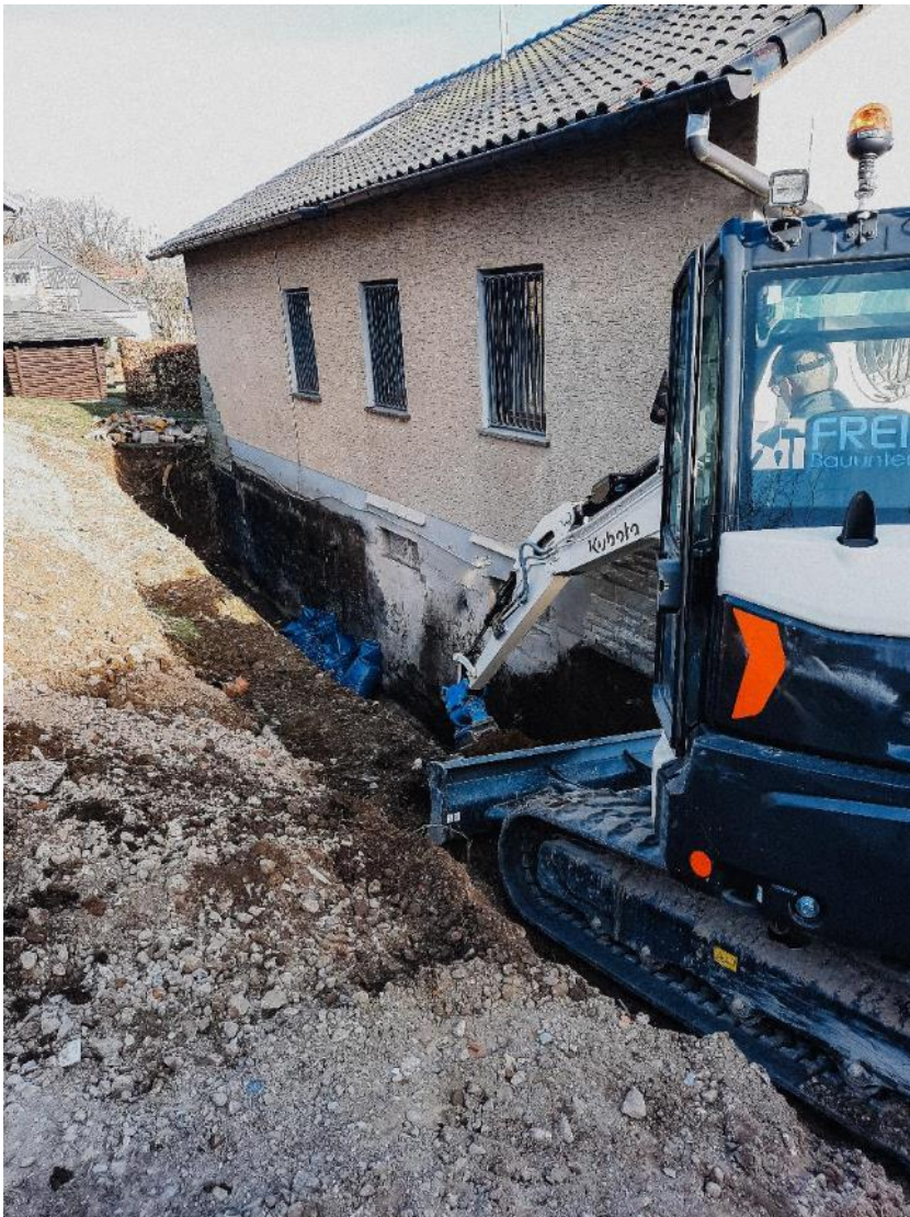
To get to the damp wall, the craftspeople exposed the basement from the outside. ( Link to high-resolution photo)
