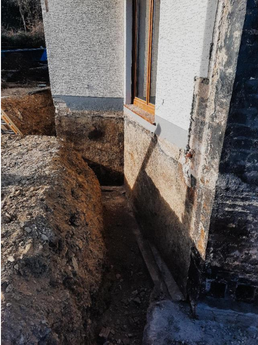
The moisture on the outer wall had to be removed as part of refurbishing the basement. ( Link to high-resolution photo)
