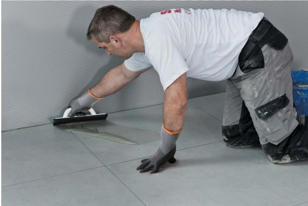
Fig. 5: The tilers used PCI Nanofug Premium for grouting the joints. This variable, flexible joint grout has a convenient working time of about 40 minutes.
